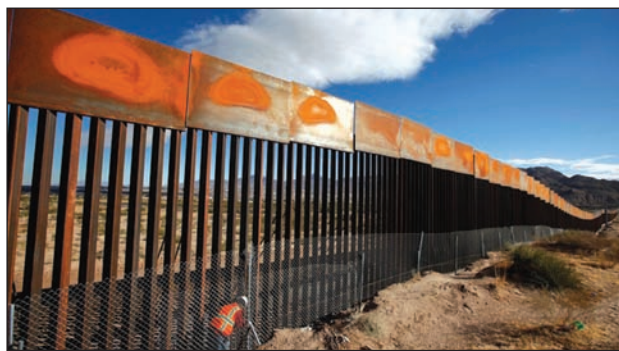
A U.S. worker inspects a section of the U.S.-Mexico border wall at Sunland Park, New Mexico.
